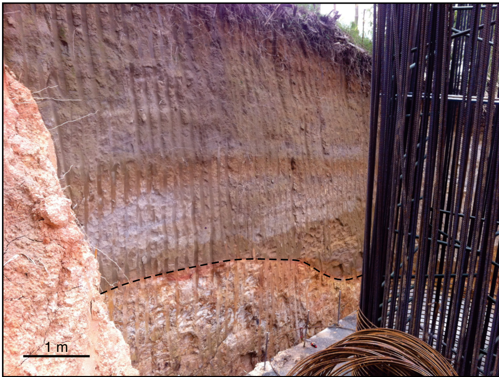
Figure 12. Sequence of redeposited volcanic ash showing subhorizontal bedding and unconformable relationship with the pre-Quaternary basement (Quebradagrande Complex). Excavation for the Intercambiador de Versalles, Calarcá, October 2016.
